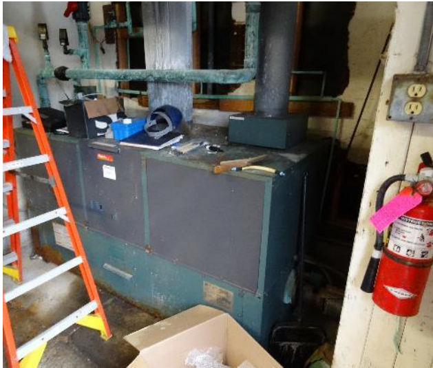
Existing Pool Boiler
